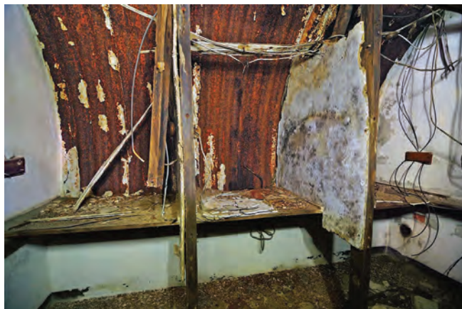
The three wireless bays. Photo Chris Warren
